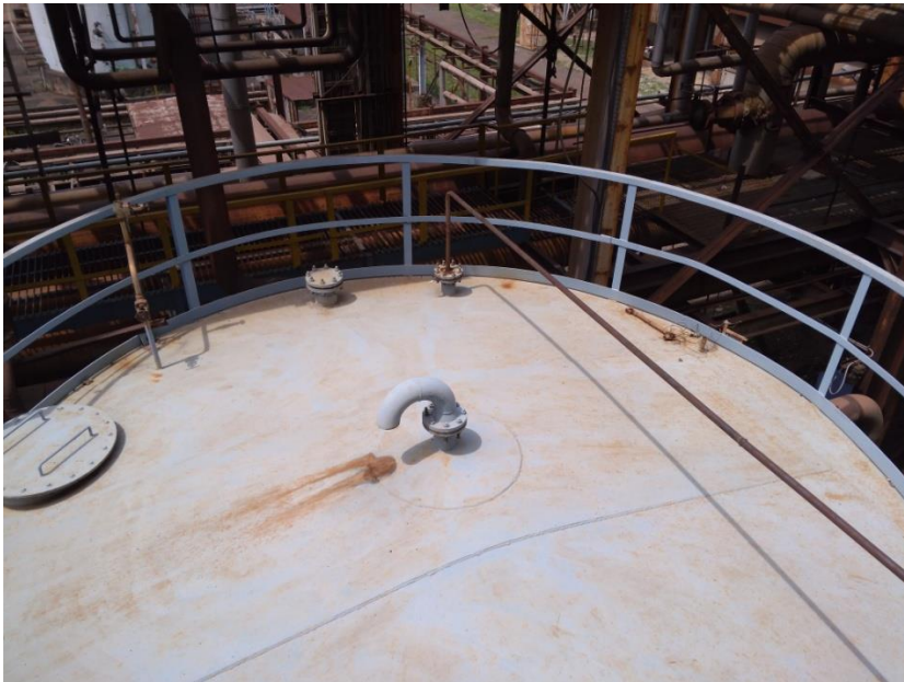
Drain line connected to condensate storage tank (CST) for recovering condensate
