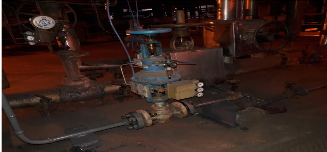
Temperature control valve (TCV) installed in drain line to control auxiliary steam temperature in auto mode
